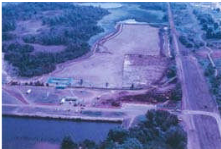
Figure 4. Hog Island Inlet is isolated to enable dry excavation of contaminated sediment.
